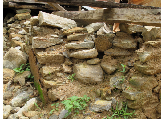
Typical mud-bonded stone wall broken up in the centre
