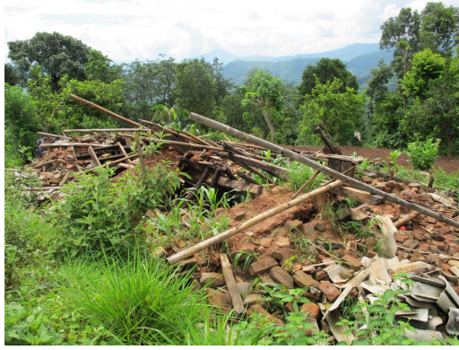
Destroyed houses with mud-bonded stone construction
