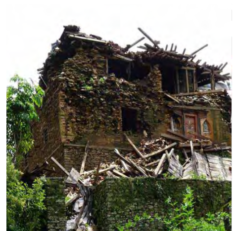
Poorly constructed stone house in the same village in Dolakha district (pictures: Dave Hodgkin, IOM)
